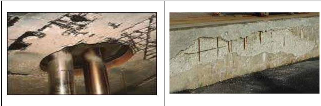
Fig 3: Spalling of concrete
